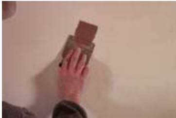
Photo 3: Putting the plaster down in an amount no larger than the square of the blade.
